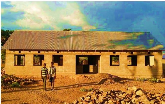
Workmen in front of the newly roofed classrooms and office block at Itumba Hill Primary School, Tanzania. SHOCC has provided funding to enable this excellent project to move towards completion.
