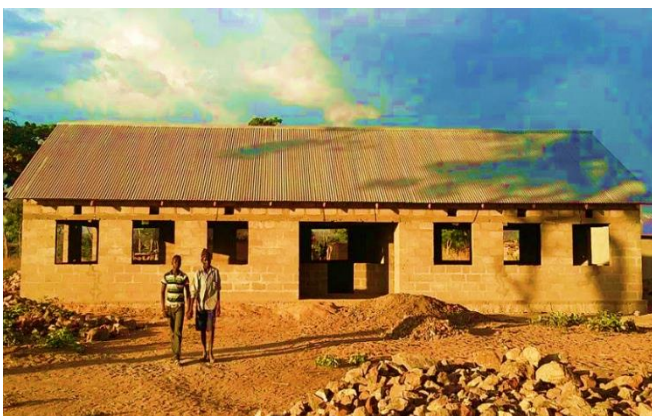
Workmen in front of the newly roofed classrooms and office block at Itumba Hill Primary School, Tanzania. SHOCC has provided funding to enable this excellent project to be completed.
