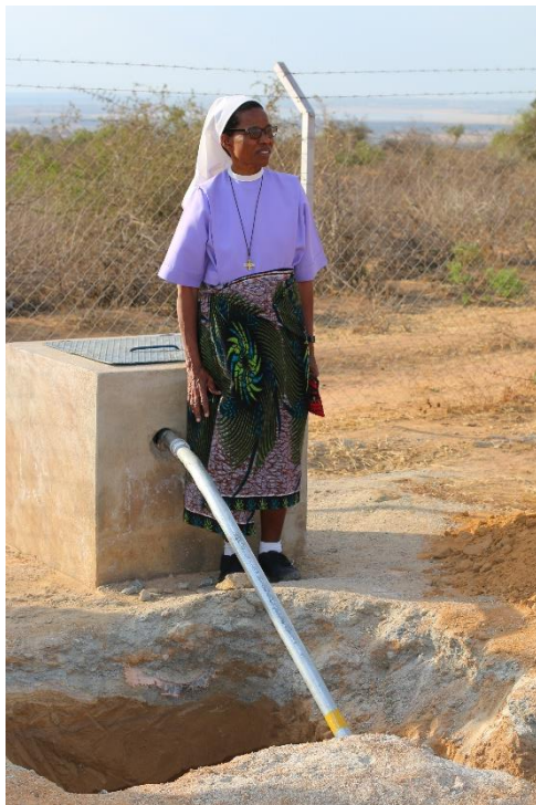
Project manager, Assumption Sister Schola, inspects the pipe that will take water from the SHOCC funded borehole to the central water tower
